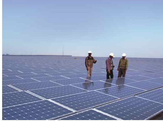
1MWp rooftop system at Thyagraja Stadium, New Delhi, India
