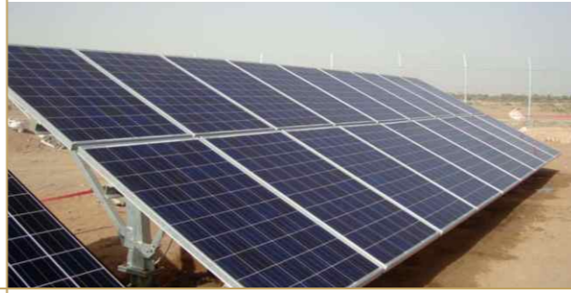
5MWp Solar PV power plant in Rajasthan
