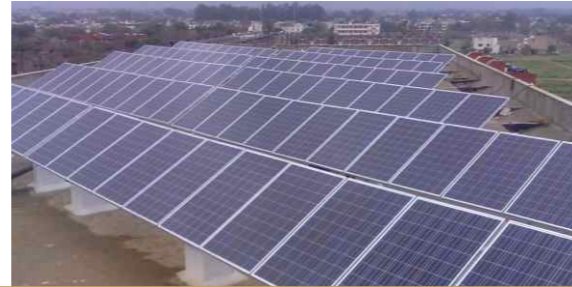
50kWp rooftop system, Chandigarh, Punjab, India
