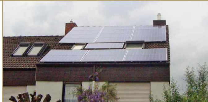
10kWp rooftop system in Germany
