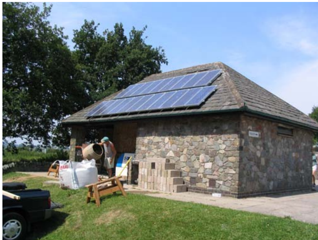
A cost effective solution - Multiple 80W solar panels installed at a park to provide lighting and automatic gate opening all year round.
